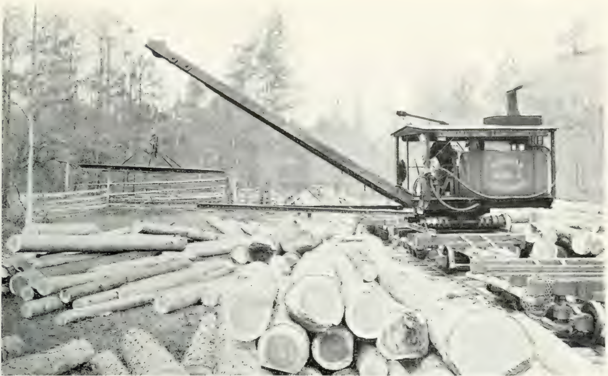
American log loader laying its own rail sections, in midst of act. American Hoist & Derrick Co., St. Paul, Minn.
