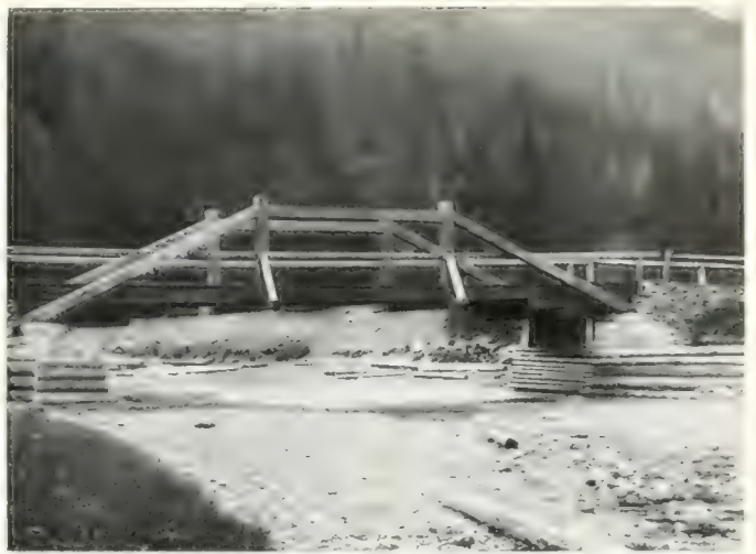
Bridge across stream used for log drives. Notice the clever combination in the bridge of bracing and suspending members.
