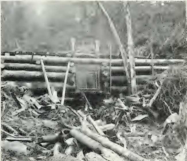
A small splash dam used for splashing of pulp-wood, Western North Carolina.
