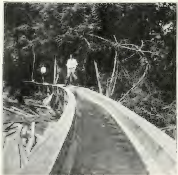
Hexagon lumber flume, near Biltmore, North Carolina.
